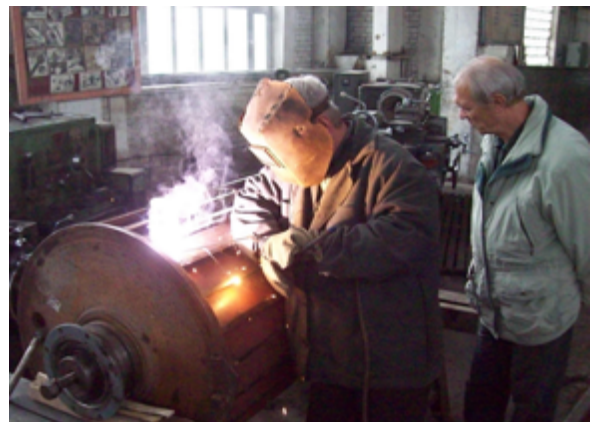
Mini hydro power plant Flickr / UNDP
